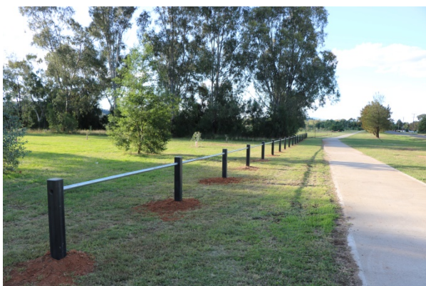
Post rail fencing installed along Wandobah Road to restrict unauthorized vehicular access
