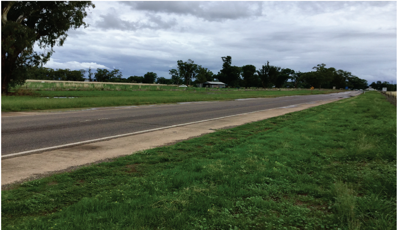
The road level of the Oxley Highway at Hoss Causeway will be raised to improve flood immunity
