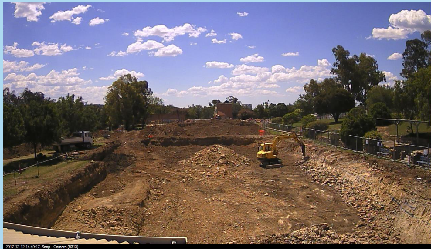
Photo: Demolition work on the Gunnedah Memorial Pool Complex as captured by the digital time-lapse camera.
