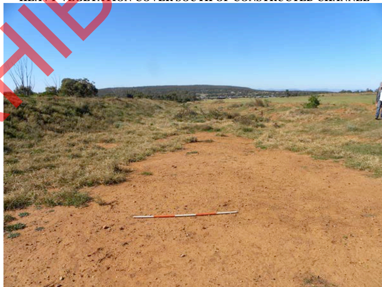
BARE PATCH IN THE CENTRE OF CONSTRUCTED CHANNEL
